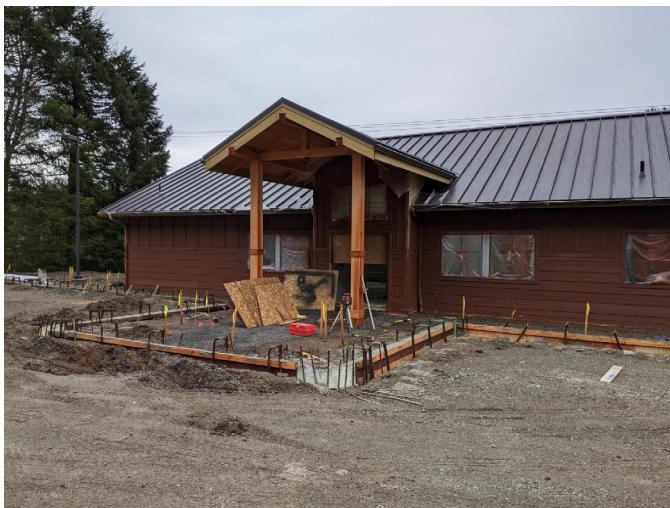
Construction of the new Ridgefield (top) and Yale Valley (below) Community Libraries will be completed in 2021.
