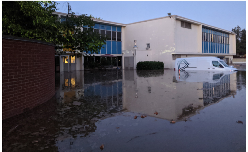
Reflected in our 2021 budget is repairs and recovery after a flood impacted our Operations Center last fall.
