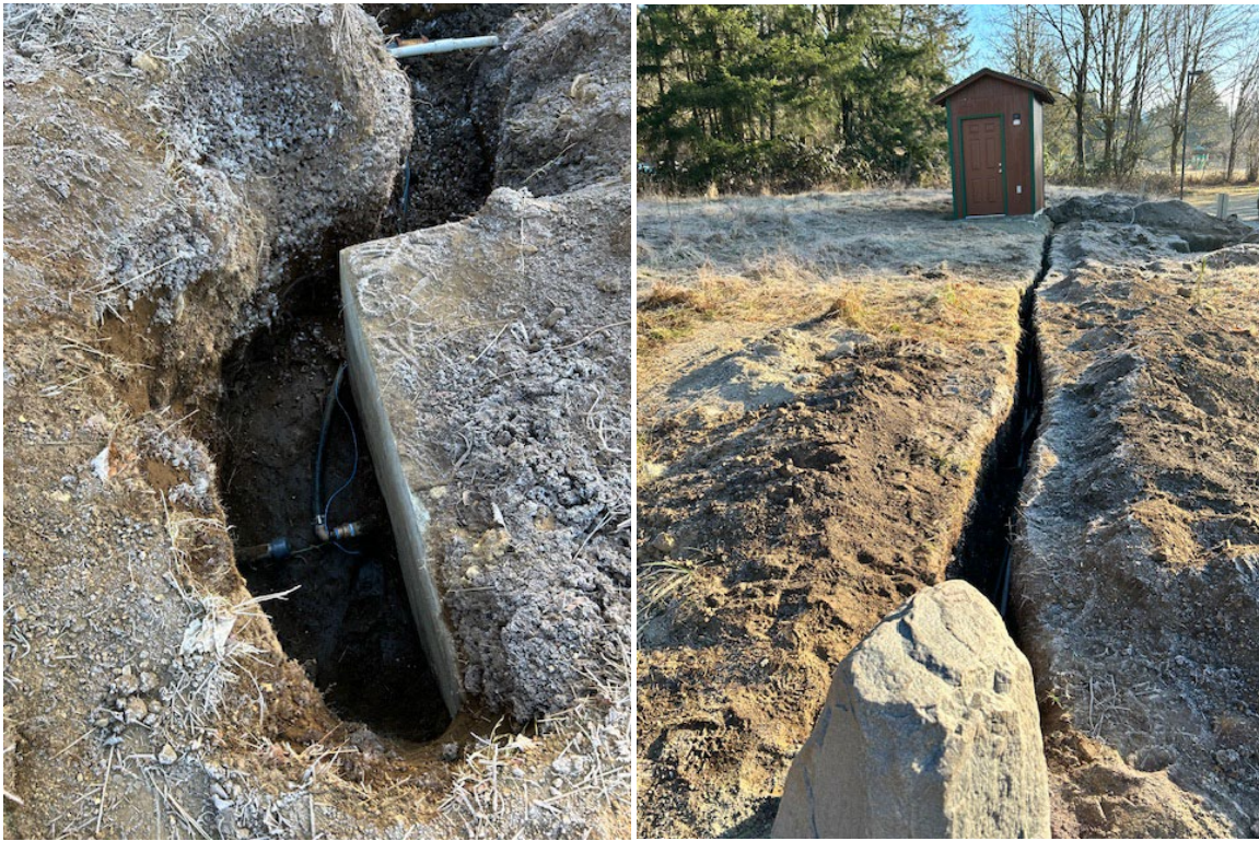
New connection to the storage tank (left); Power and water-line to the pump house (right)
